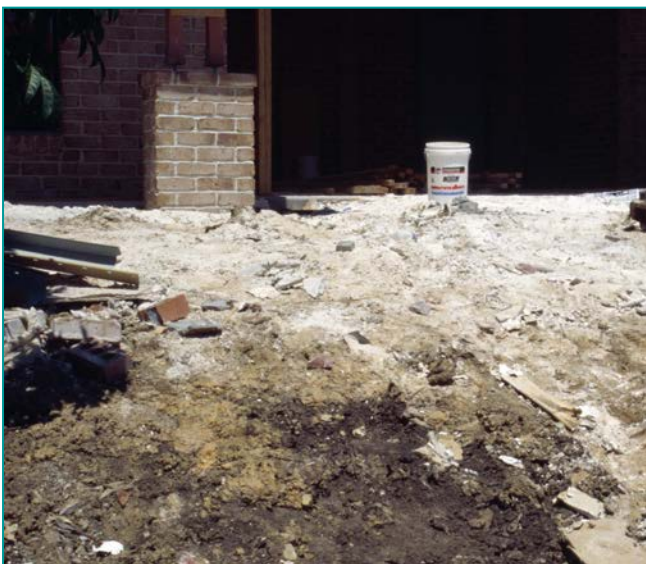
Plaster & builders rubbish contaminates soil
