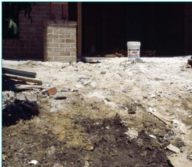
Plaster & builders rubbish contaminates soil
