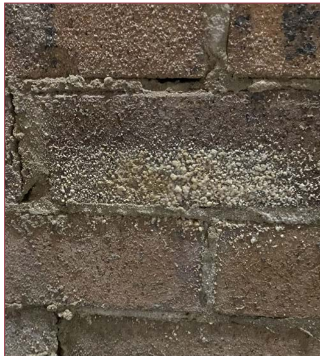
Poor drainage behind a brick wall can be indicated by salt deposits left behind by salty water seeping through the wall.
